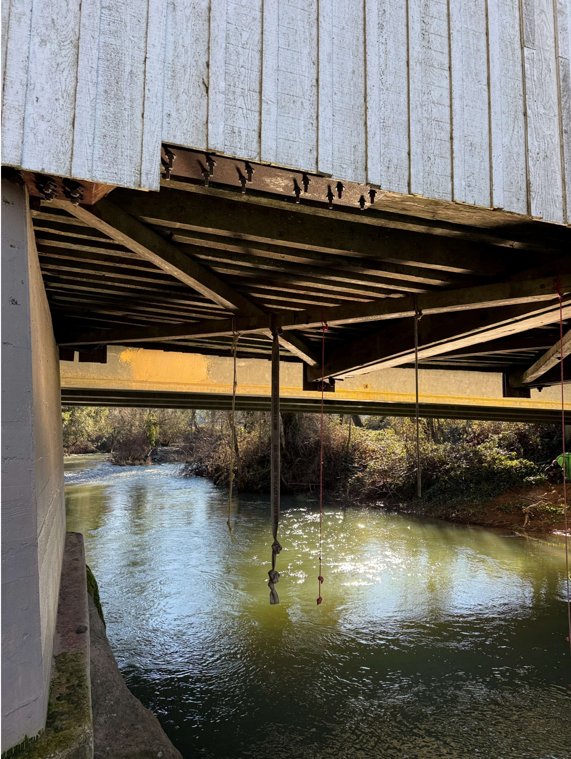
Figure B3: Stewart Bridge: Downward deflection at floorbeam 3
