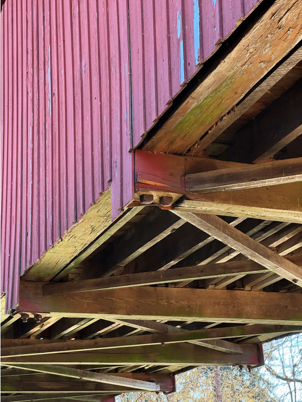
Figure B4: Currin Bridge: Crushing at floorbeam 6 east
