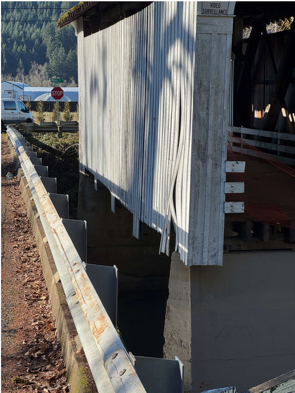
Figure B1: Stewart Bridge: Siding Buckling Bent 4 SE Corner
