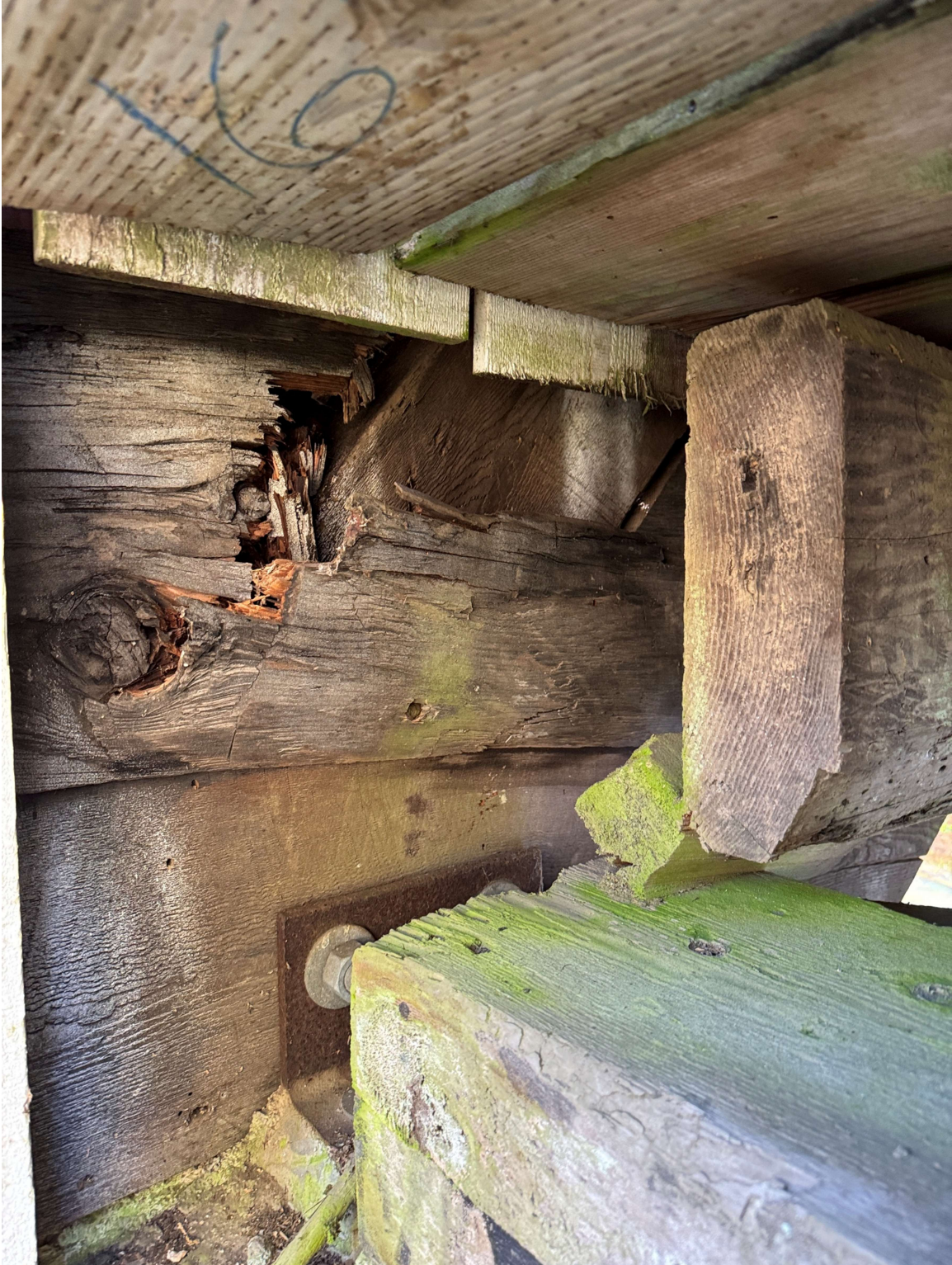
Figure B2: Stewart Bridge: Crushing at Right Truss Bottom Chord (Bent 4)
