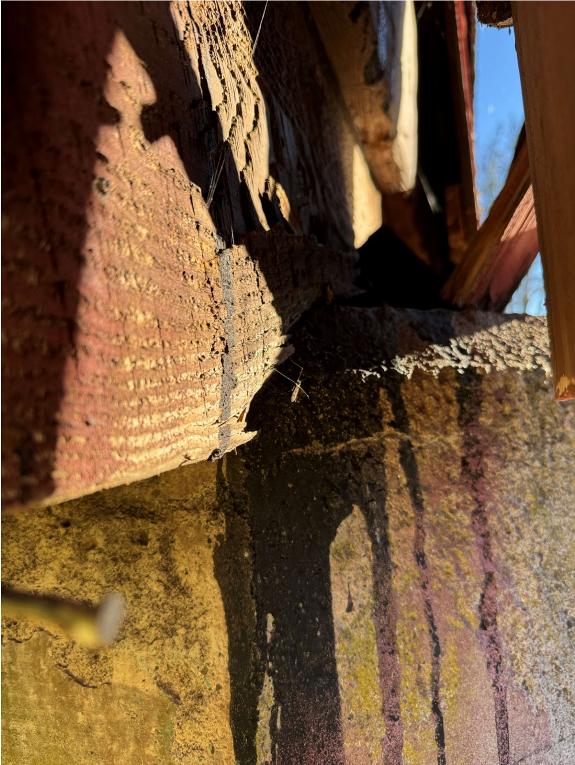
Figure B5: Currin Bridge: Crushing at Bent 6 West Corbel
