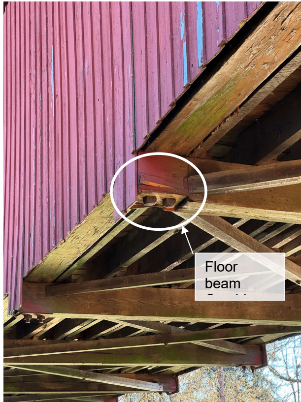
Figure 2: Floor beam Crushing and Shearing at Hanger Rod Connection
